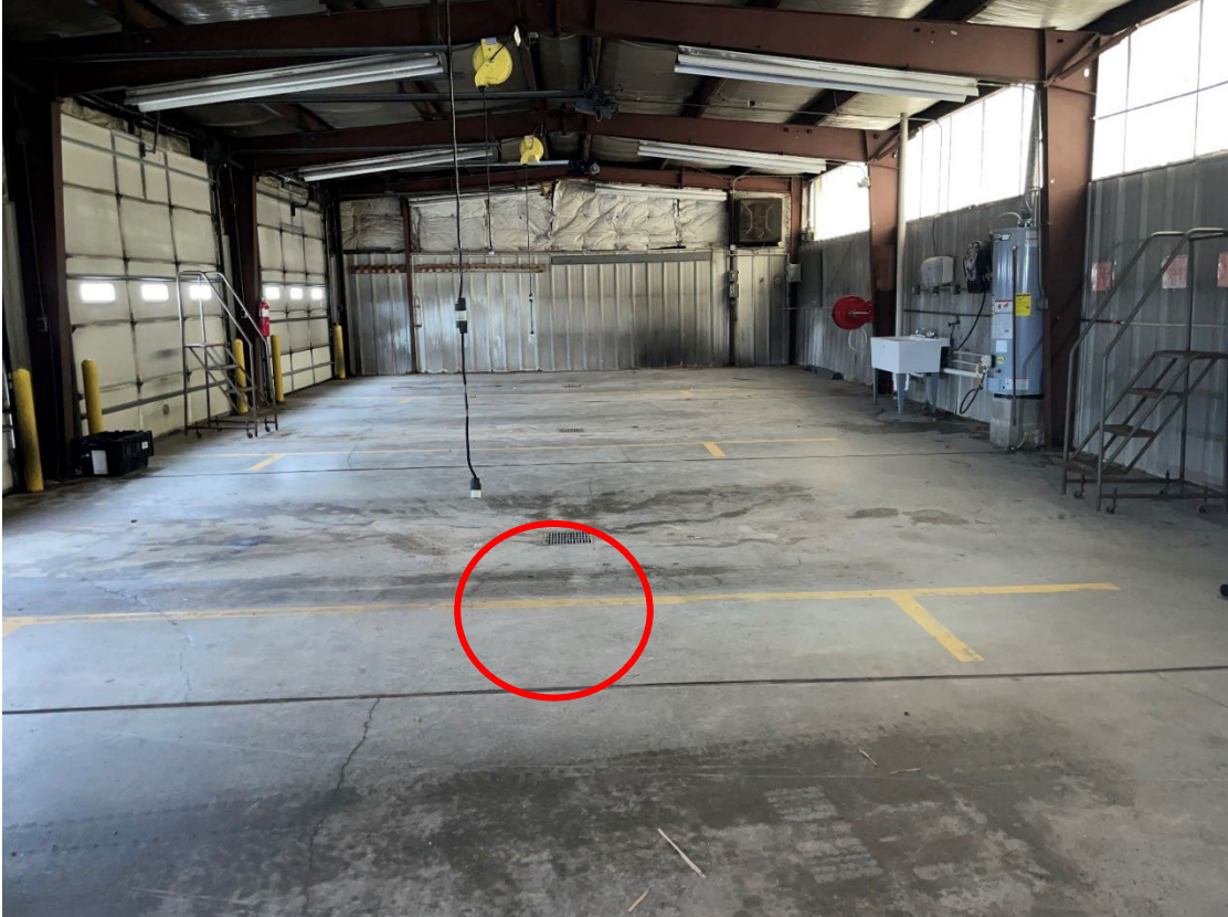
Photo 13: Subject Site – Floor drains in auto repair bays in ambulance repair shop.
