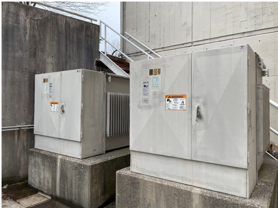
Photo 10: Subject Site – Pad-mounted transformers south of 714 S. Rogers, nursing home.
