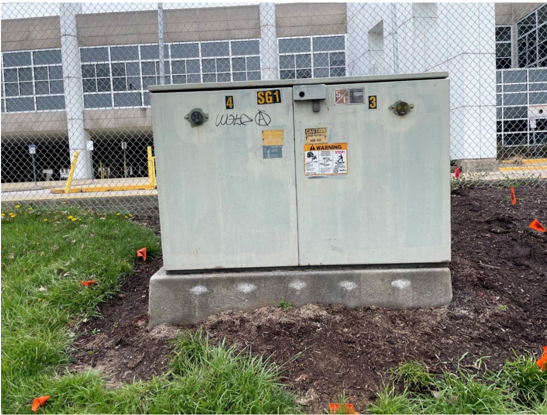
Photo 18: Pad-mounted transformer on adjacent property to the north of the Subject Site.
