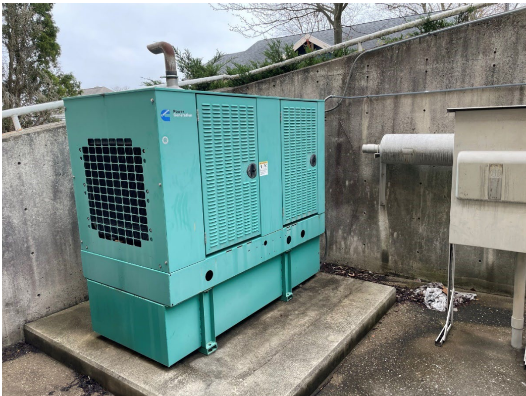
Photo 8: Subject Site – Generator with fuel tank south of 714 S. Rogers, nursing home.
