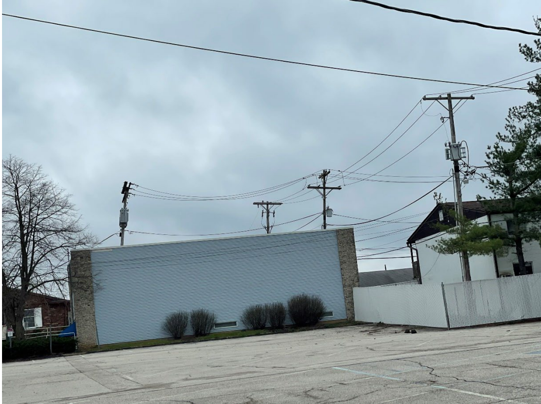
Photo 9: Subject Site – Multiple pole-mounted transformers.
