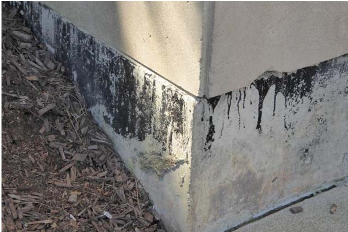
Photo 46 The original bitumen based waterproofing has deteriorated badly.
