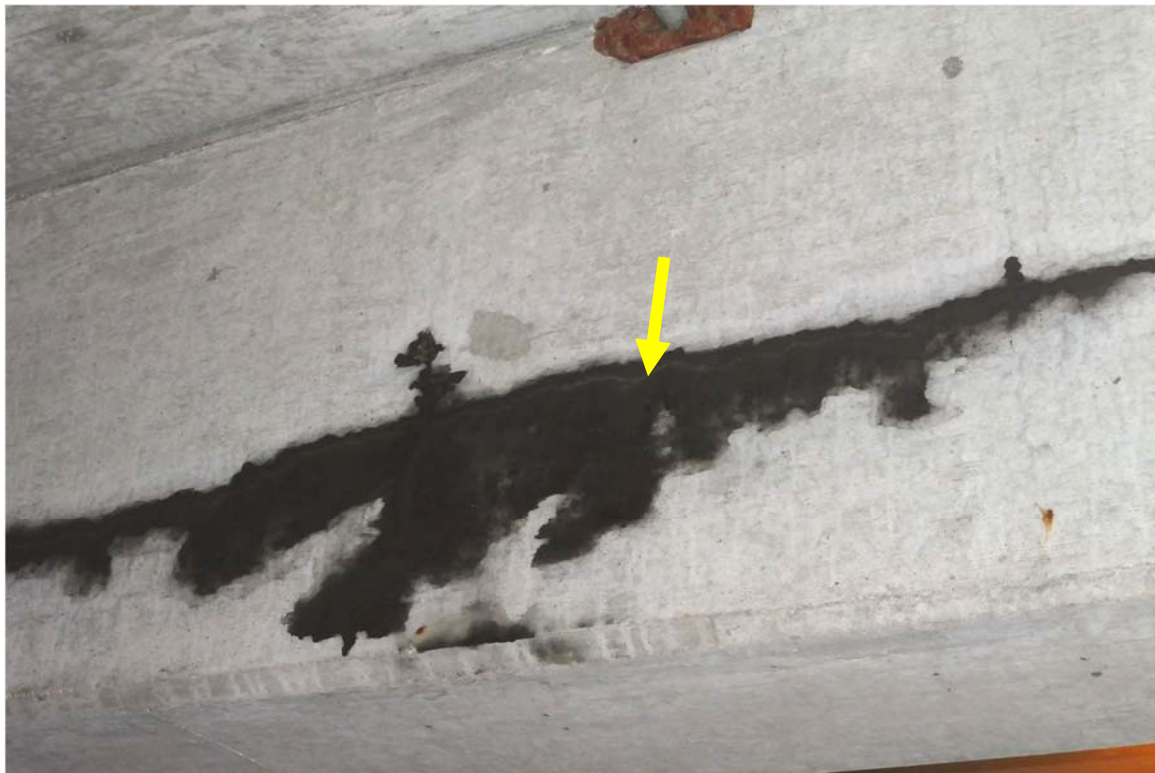
Photo 66 Close-up view of Photo 7. Note the crack seen through the grease staining.
