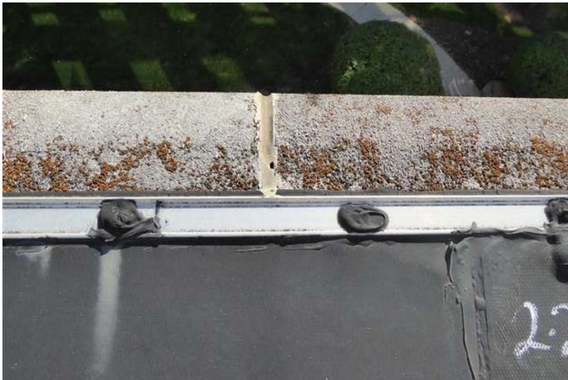
Photo 14 The membrane turns up over the back and top of the limestone coping and is secured with a termination bar.
