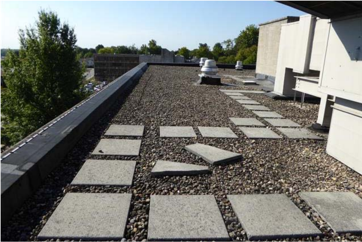
Photo 13 The roof is covered with a ballasted EPDM. The roof is reported to be at least 30 years old.
