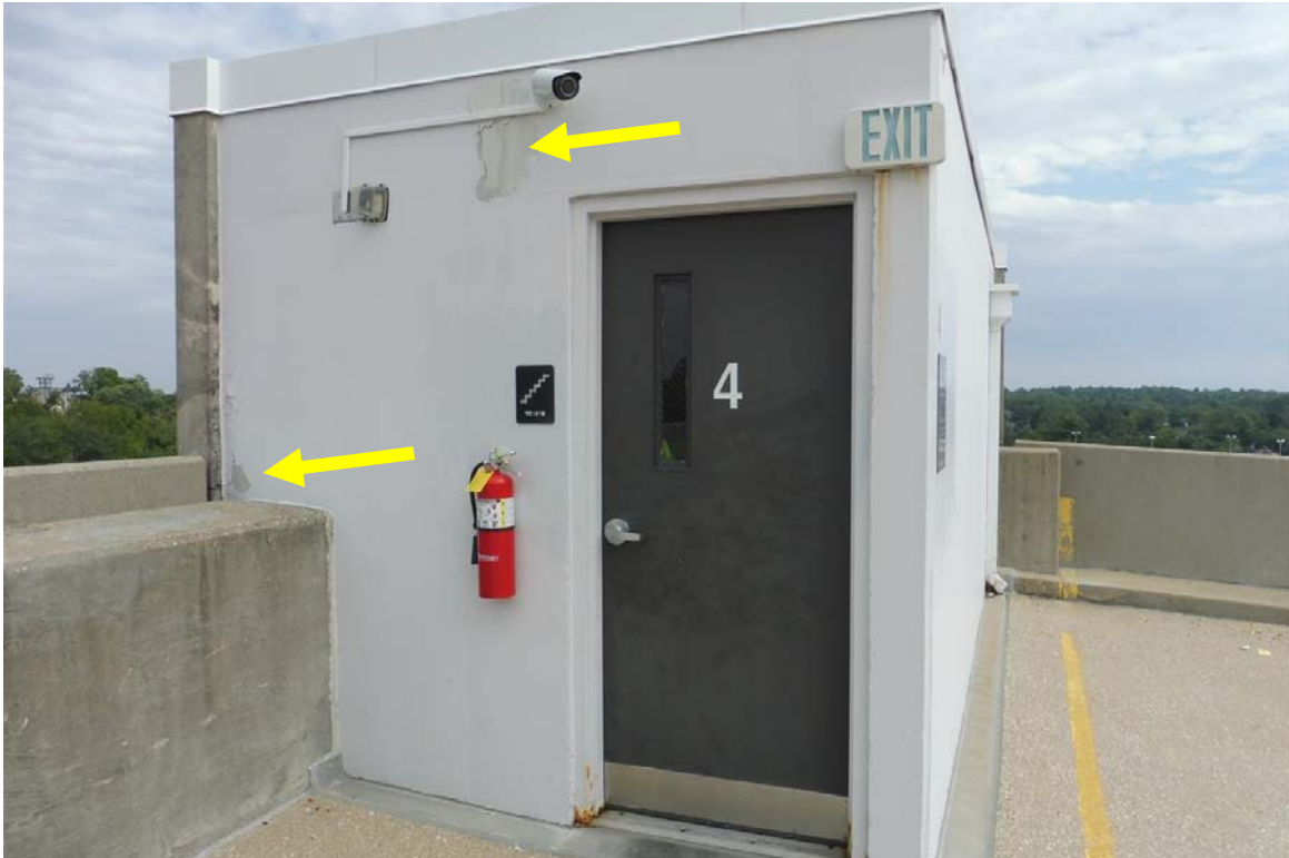
Photo 111 Northeast stair tower at the roof level. The coating on the concrete walls has failed in multiple areas on the outside of the stair tower.
