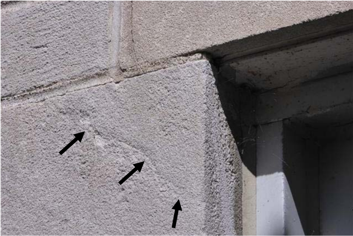
Photo 31 A cementitious patch was installed at a previous spall.
