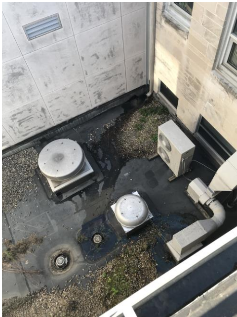
Heat pump, on right
