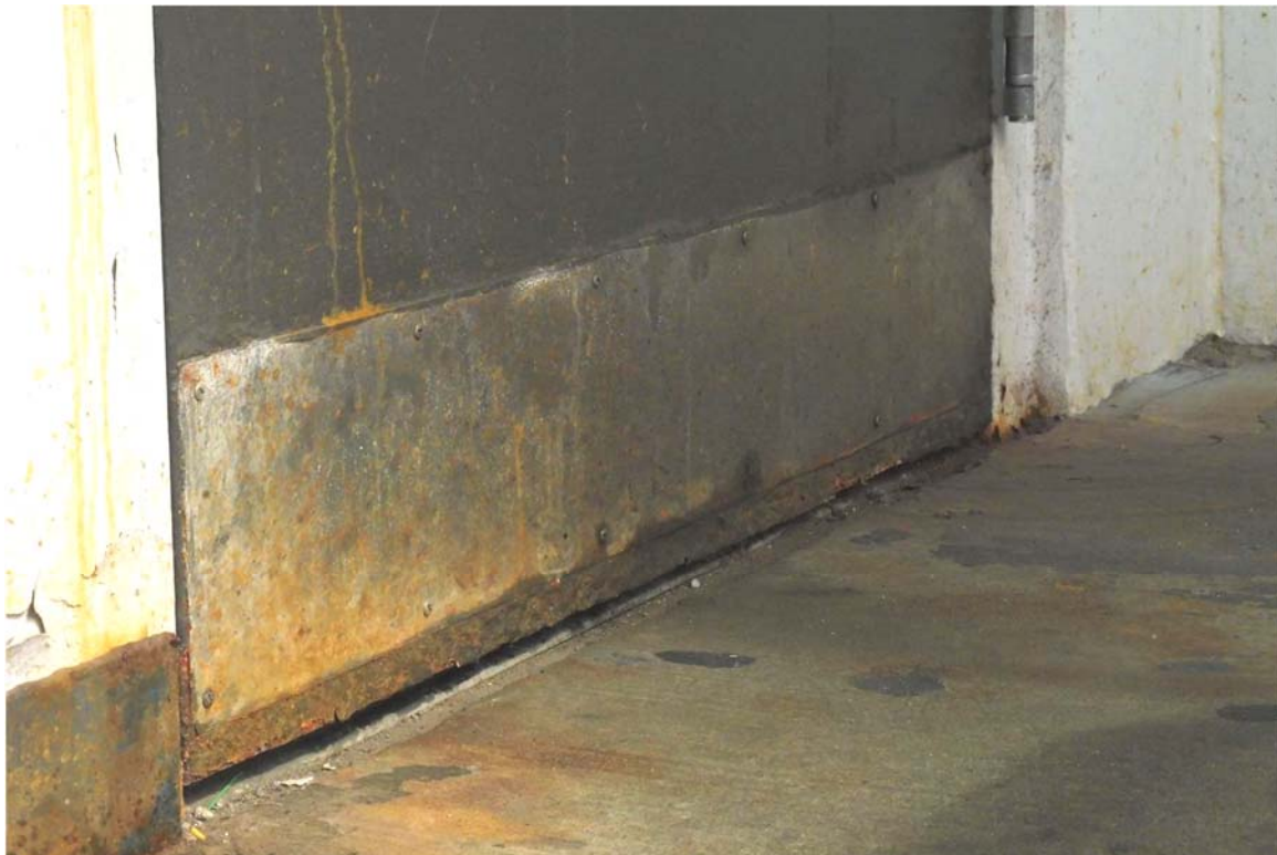
Photo 104 ...as well as the hollow metal doors was observed on each level of the southwest stair. Regular maintenance of the coatings on the doors and frames will help minimize the corrosion levels.
