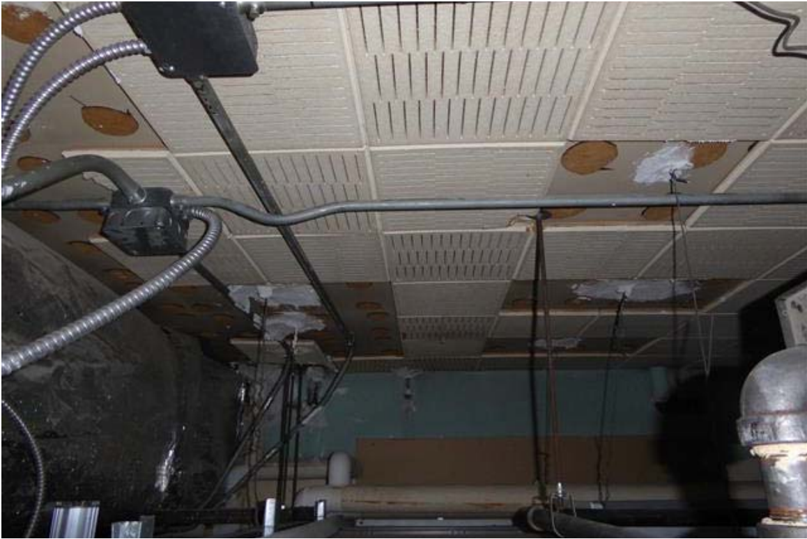
Photo 53 Typical view above the drop ceiling. The original glue on ceiling tile and plaster ceilings are still in place.
