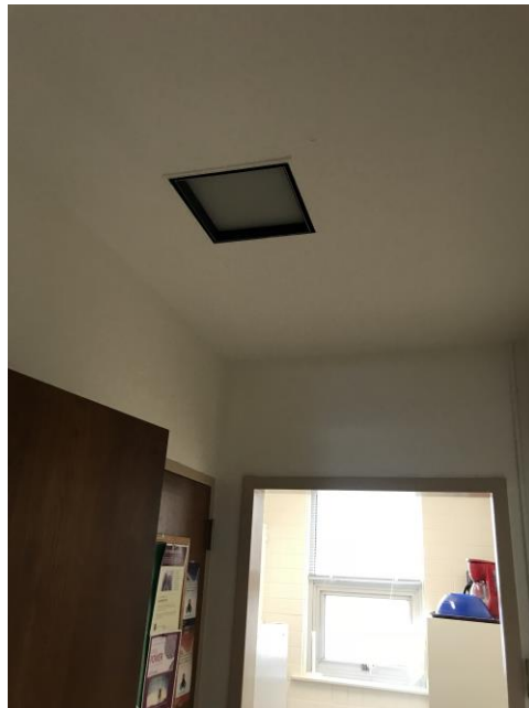
Typical recessed downlight
