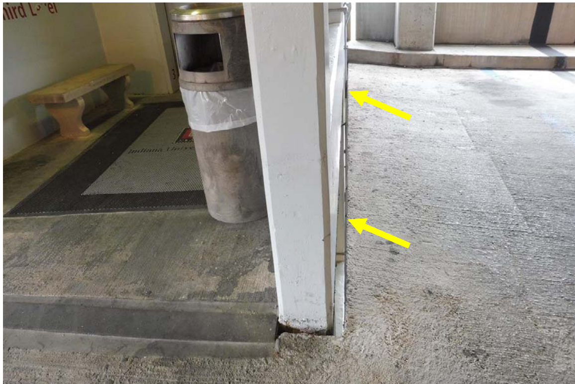
Photo 110 The expansion joint between the southwest stair/elevator tower and the garage floor slab is open at Levels 2 and 3. We would suggest an expansion joint be installed to seal the gap.
