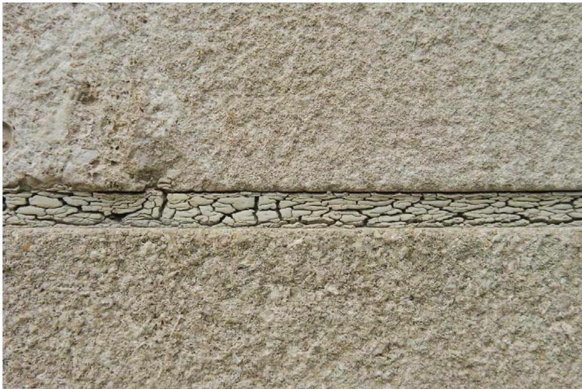
Photo 86 ...have reached their useful service life and should be replaced.
