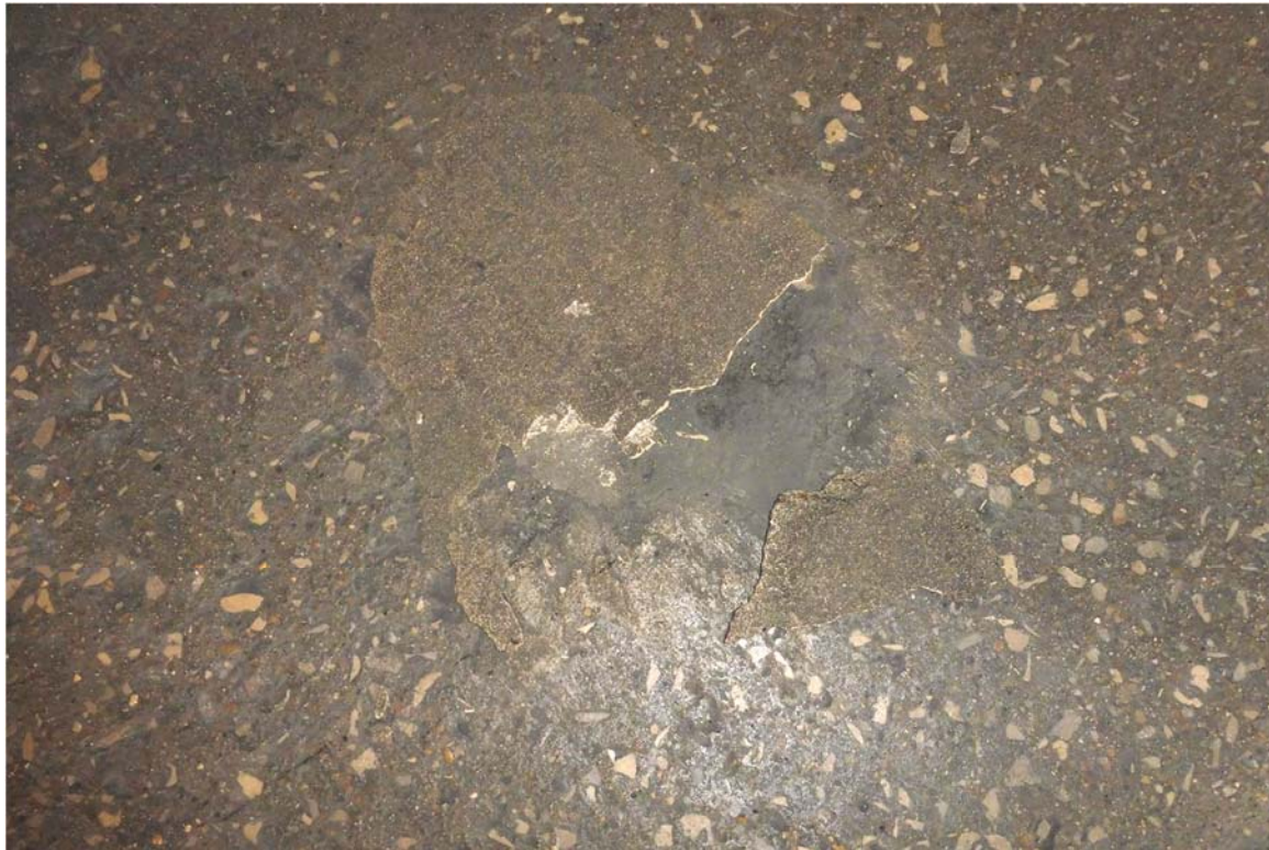
Photo 76 Another example of surface scaling that was observed.
