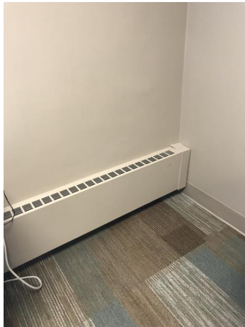
Perimeter hot water heater
