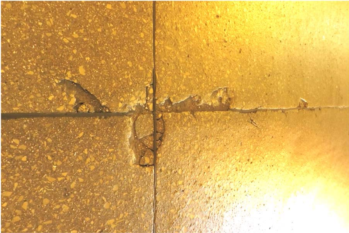
Photo 77 Small spalls in the slab-on-grade at the sawcut control joints should be patched to keep from enlarging with time.
