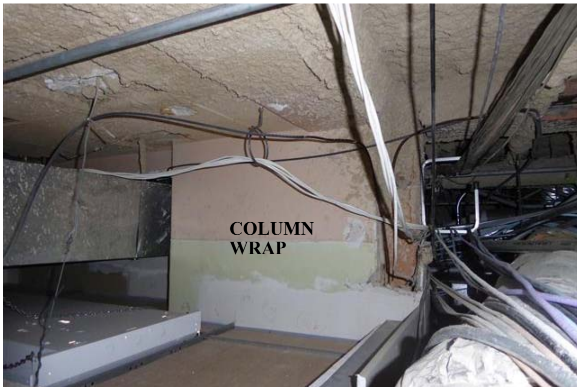
Photo 54 Steel framing supports the second floor, third floor and roof levels. The steel columns are wrapped with clay tile and plaster for fire protection.
