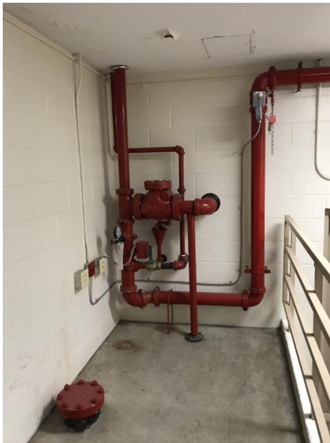
Fire riser with abandoned source line in the foreground
