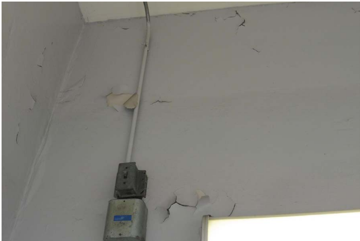
Photo 108 Example of the peeling and failed coating on the concrete walls within the southwest stair.
