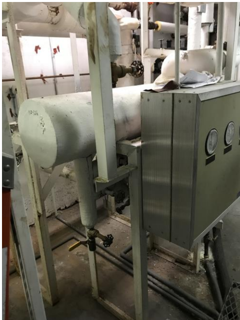
Steam-to-Hot Water Heat exchanger
