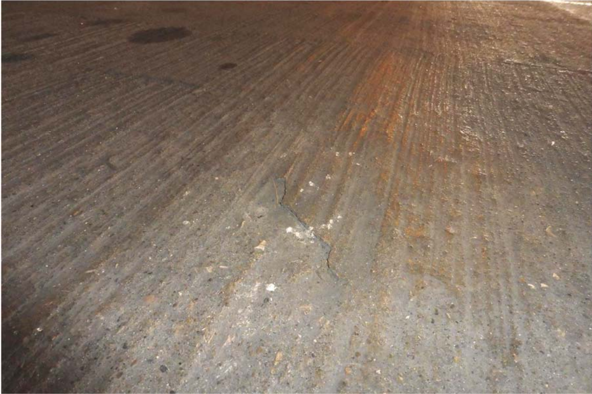
Photo 75 Slab scaling of the top surface was noted at some locations, generally on the lower levels where the volume of vehicles is typically higher.
