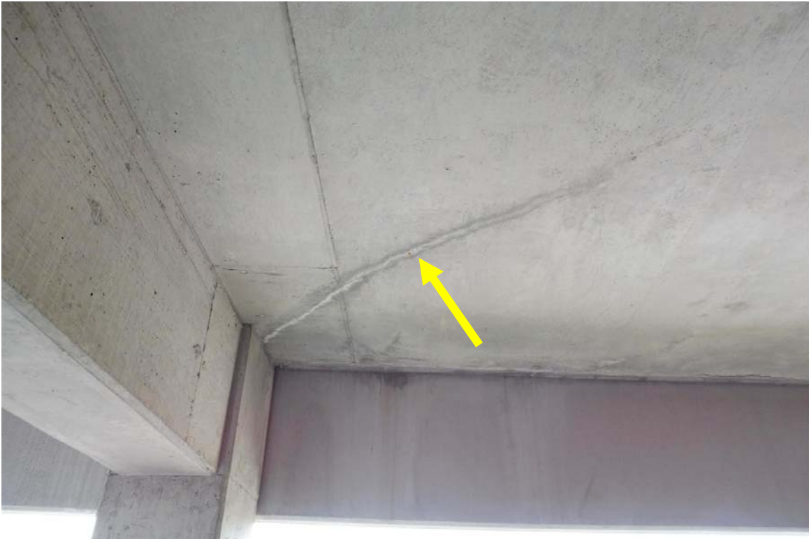
Photo 73 Cracks on the underside of the post-tensioned floor slabs existed in localized areas. The white staining seen along the crack is the result of calcium deposits on the surface from water migration through the crack.
