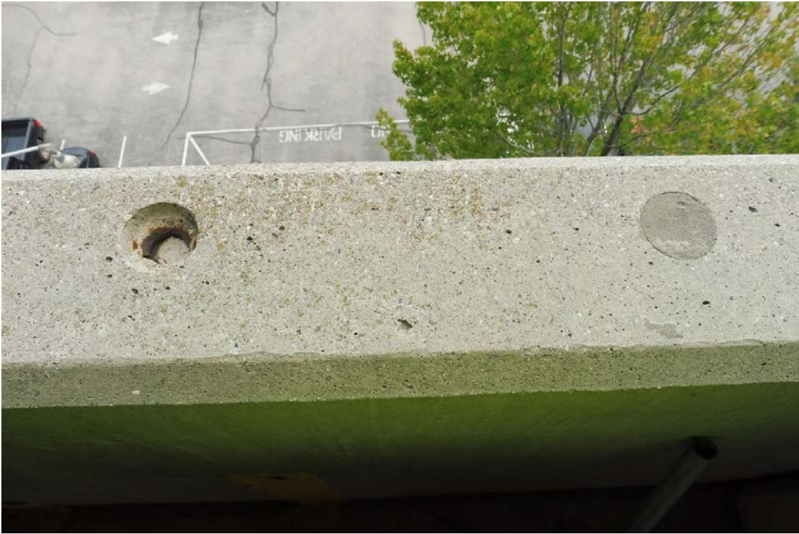
Photo 87 Missing grout pockets at the lift insert holes on the skyward face of the façade panels...
