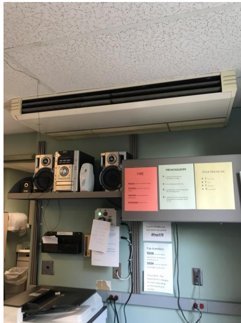
Indoor fan-coil for heat pump
