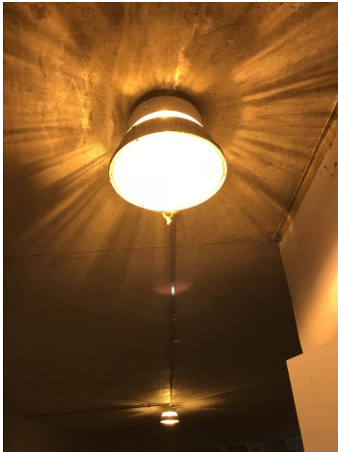
Interior garage fixtures
