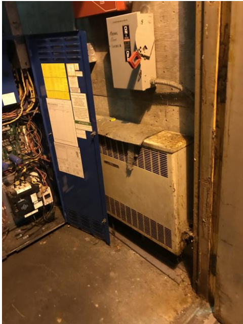
Elevator machine room heater
